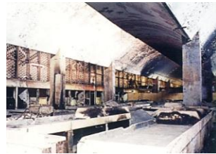
Daños a la Nave Mayor Interior
