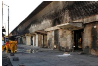
Daños a la Nave Mayor Exterior
